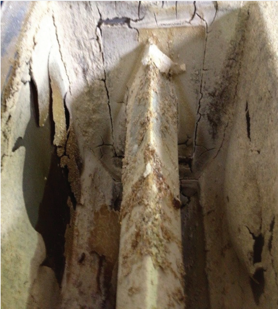
Figure 6: Surge bin with potential contamination
