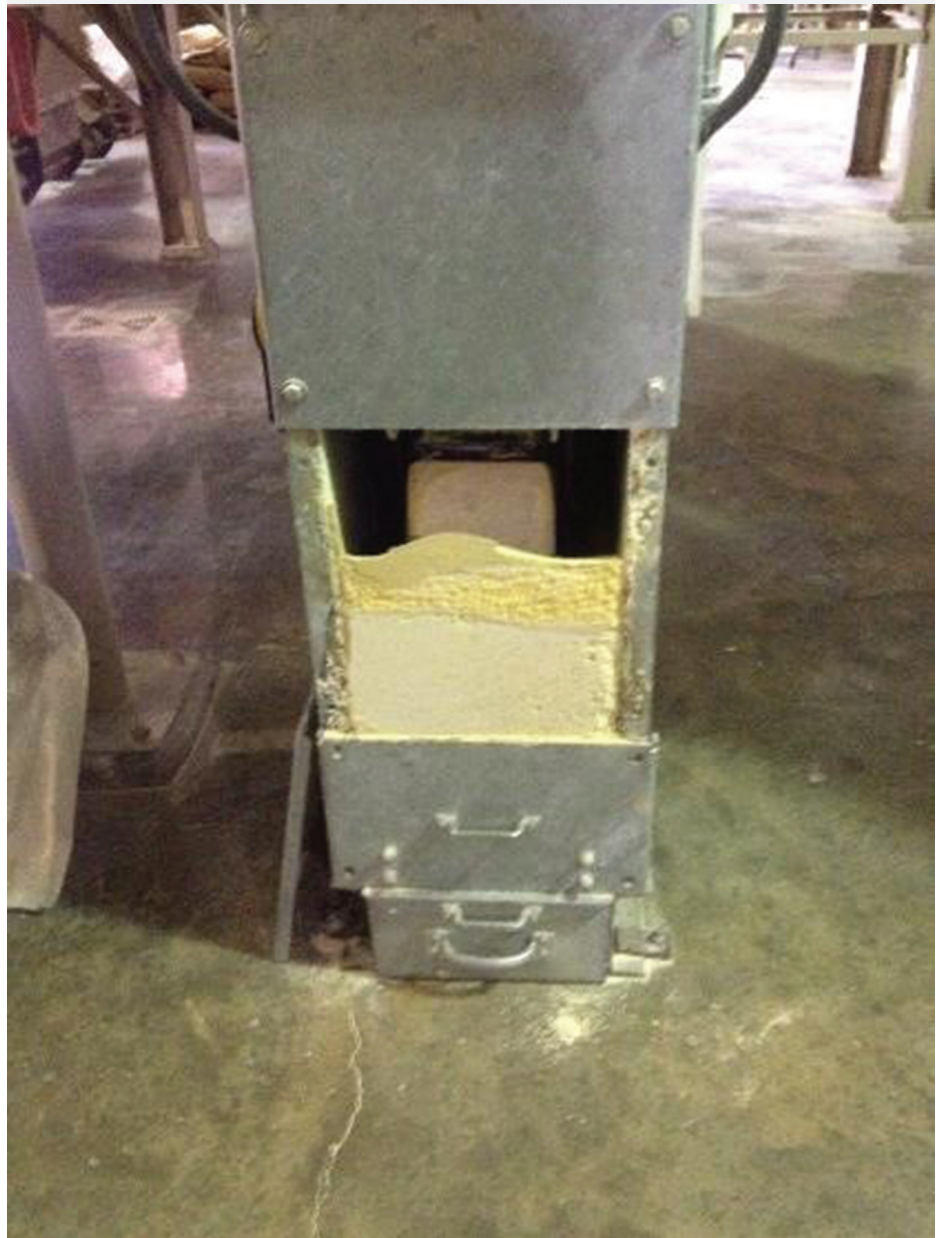
Figure 7: Bucket elevator with potential contamination
